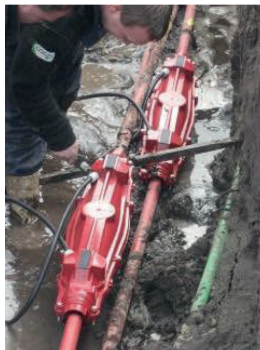
FIG. 6 Example of cross-bonding retrofitting on MV joints already in service, black bonding wires are visible
