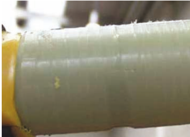
Figure 30 – Extremely rough insulation surface resulting from incorrect setting and/or misuse of screen removal tool
