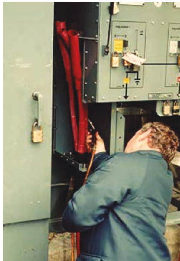
Figure 14 – Inadequate installation space between substation equipment
