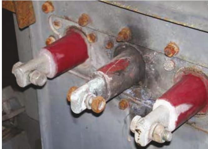
Figure 51 – Failure of a switchgear bushing after long-term partial discharge activity
