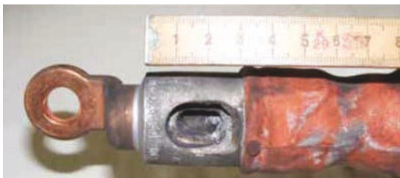
Figure 50 – Incomplete coverage of termination lug possibly allowing moisture entry
