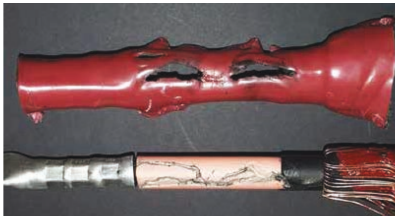
Figure 49 – Failure of a termination due to electrical tracking on the insulation surface
