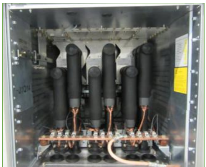
Figure 17: Double cable connection: Screened separable connectors on Interface C bushing and coupling connector in switchgear with 2 bushings for each phase, cable fixing beneath the compartment
