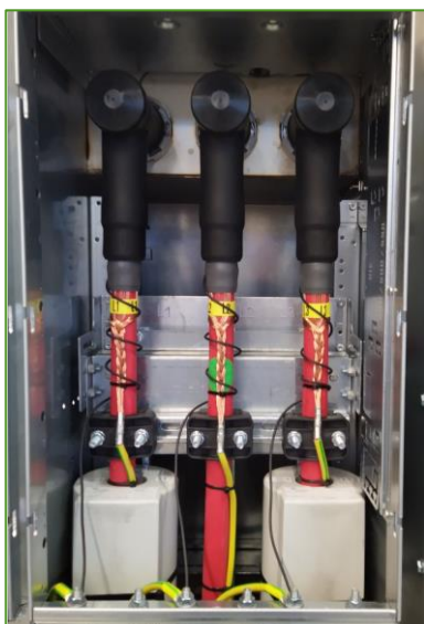
Figure 16: Cable connection in the cable compartment of a gas insulated switchgear
